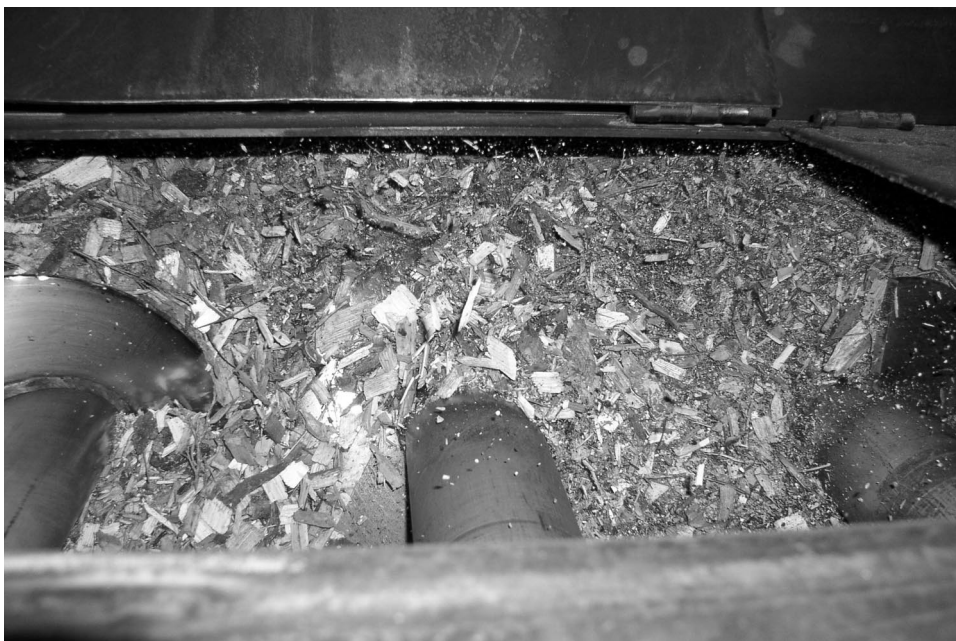
Figure 3: Wood Chips Being Conveyed to a Boiler, California Power Plant
