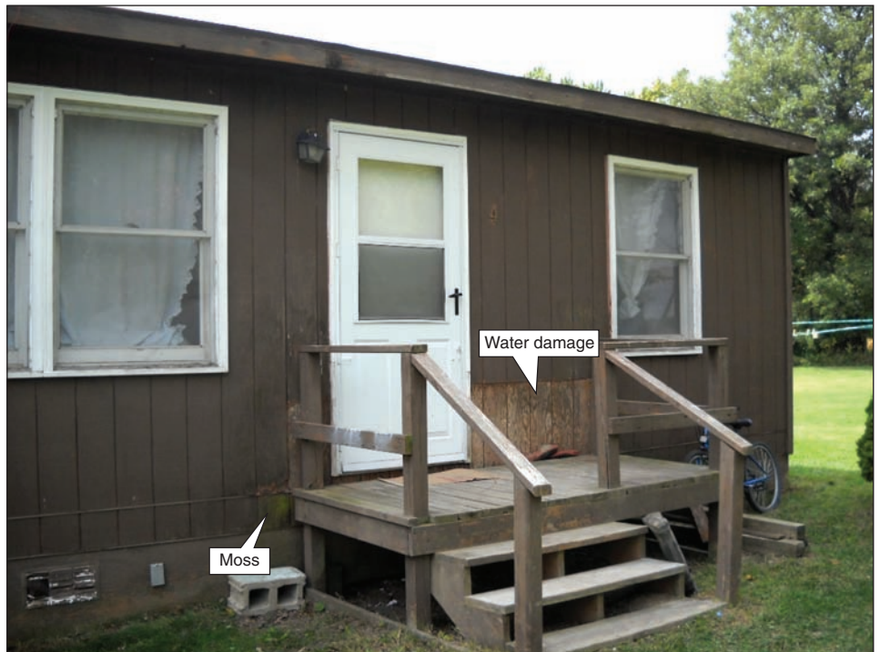
Figure 13: FLH Unit in Michigan with Water Damage to the Exterior
