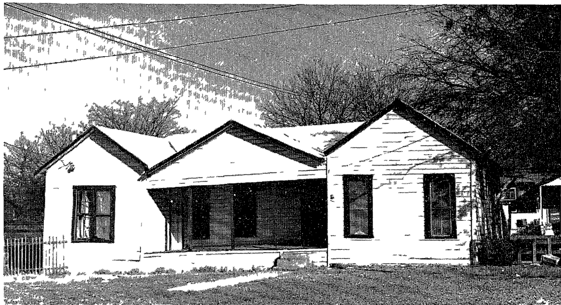
FORT HOOD, TEXAS SUBSTANDARD UNIT BECAUSE OF POOR STRUCTURAL CONDITION, WALLS, FLOORS, WINDOWS AND DOORS NEED REPAIRS
