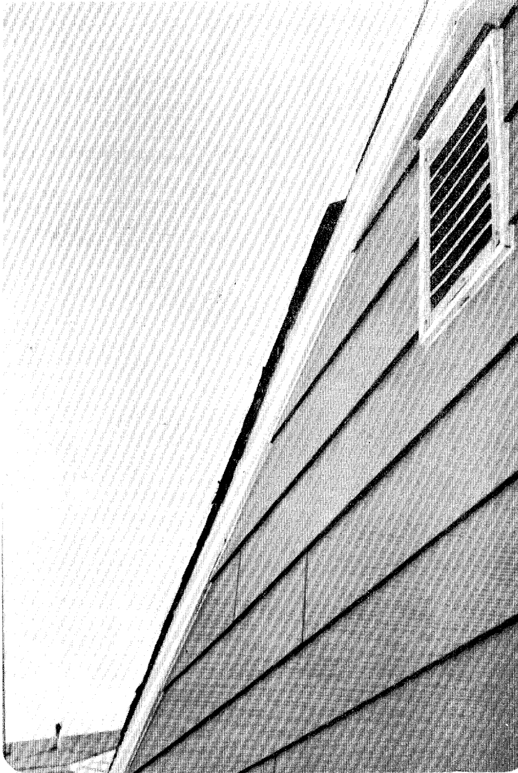
FIGURE 5 EXAMPLE OF ROOFING SHINGLES NOT OVERLAPPING EDGES OF SOME ROOFS ON NEW GARAGES.
