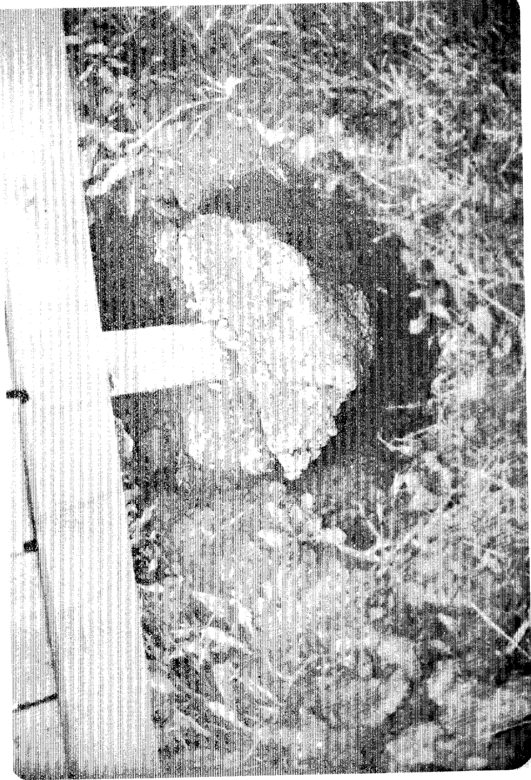
FIGURE 9 INADEQUATE ANCHORING OF FENCEPOSTS WHICH CAUSED FENCES TO LEAN.
