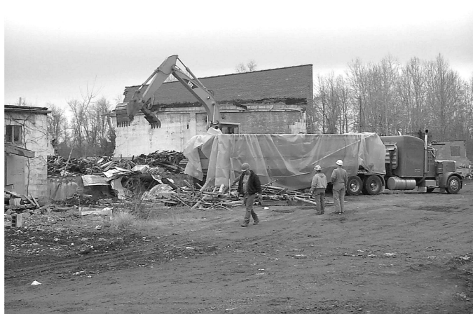
Unsafe buildings, structures, or debris
