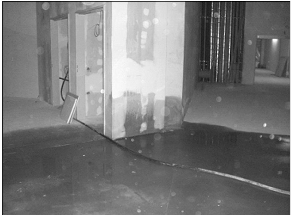
Figure 2: KMCC Damage from Leaks in Roof
