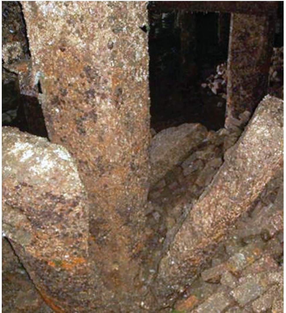
Figure 4: Deteriorated Piles under Pier 4 at Puget Sound Naval Shipyard
