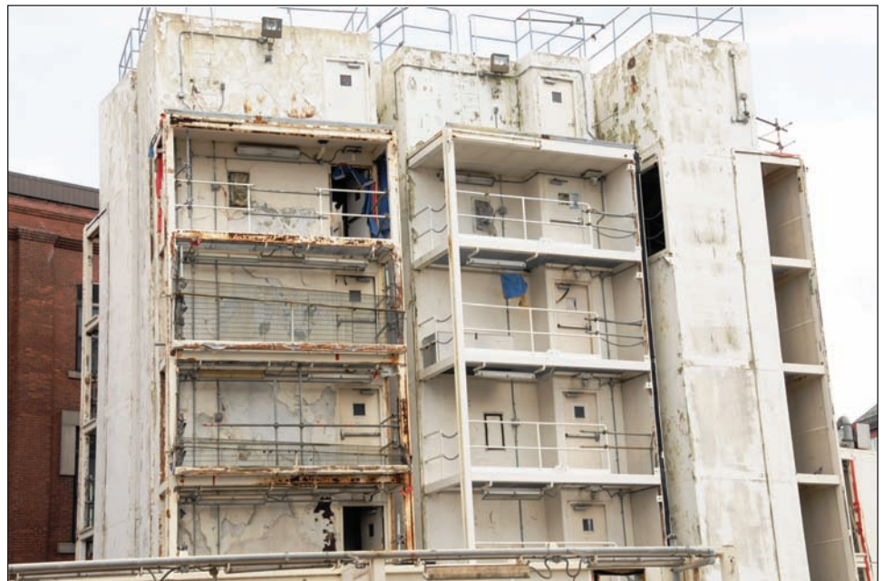
Figure 6: Rusted Movable Submarine Maintenance Enclosures at Portsmouth Naval Shipyard
