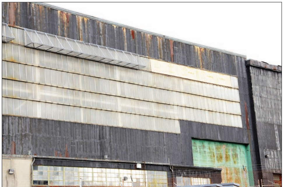
Figure 5: Broken Glass Windows Replaced by Plywood Boards at Portsmouth Naval Shipyard
