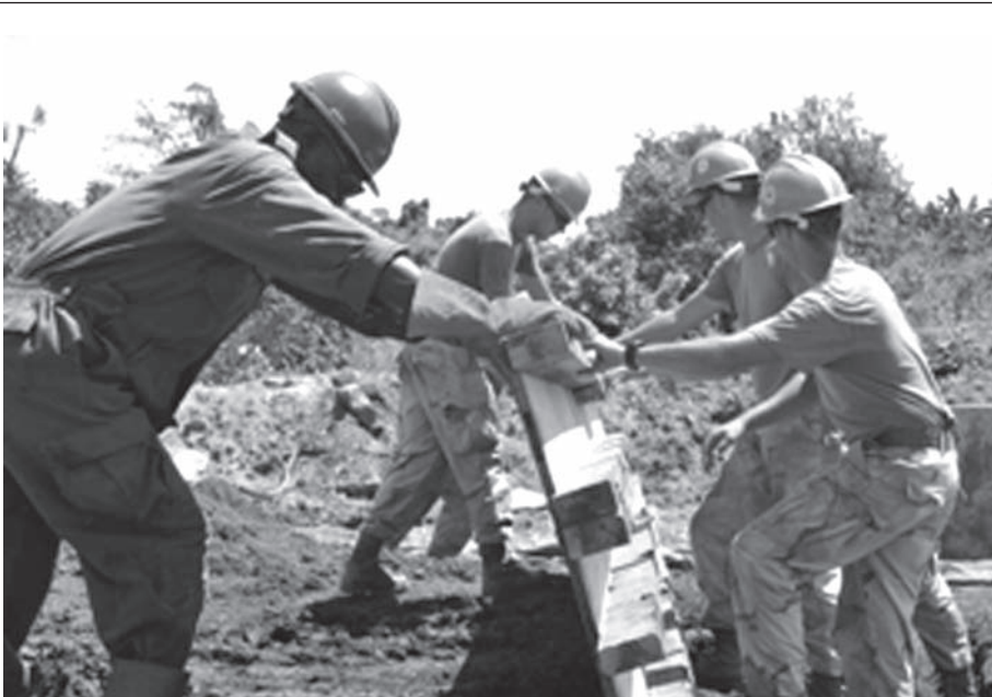
CJTF-HOA and Uganda People's Defense Force work to construct a bridge foundation
