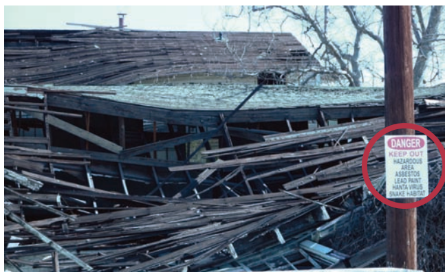
Condemned building with danger sign
