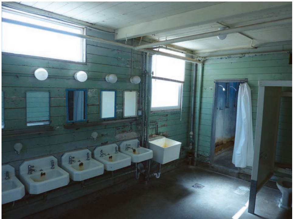
Figure 10: Unrenovated World War II-Era Temporary Building Bathroom Currently Being Used at Camp Roberts
