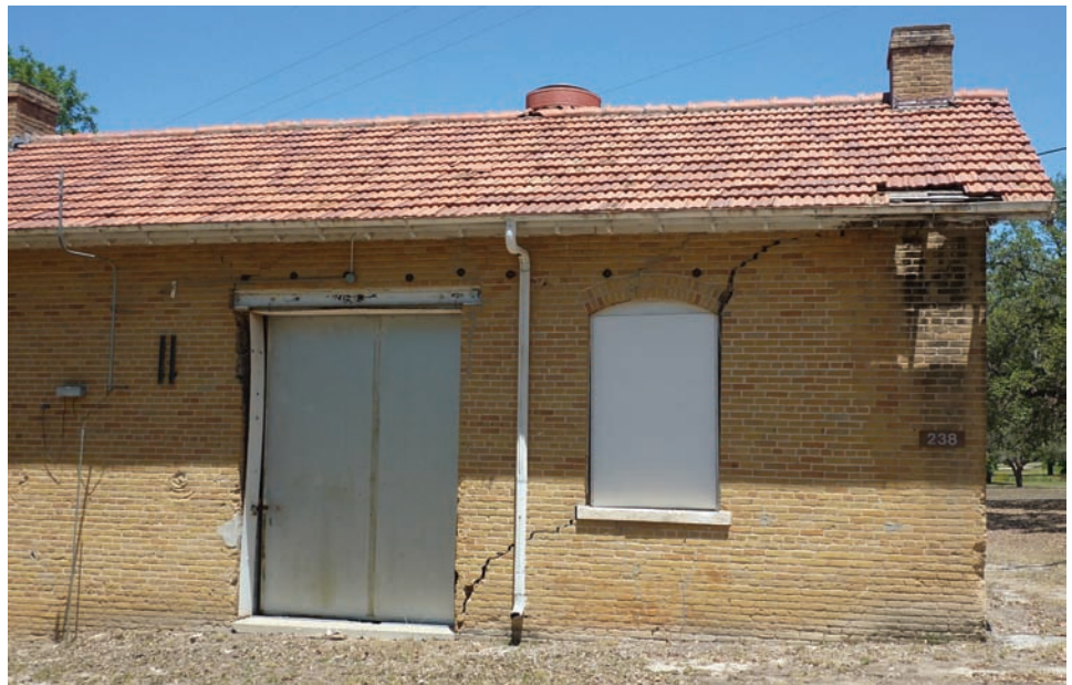
Figure 6: Historic Building 238 with Structural Cracks at Fort Sam Houston
