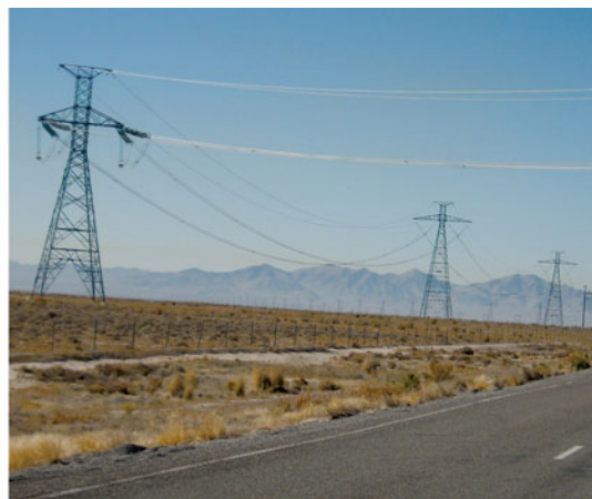
Figure 1: HVDC Transmission Line along Utah State Highway 174
