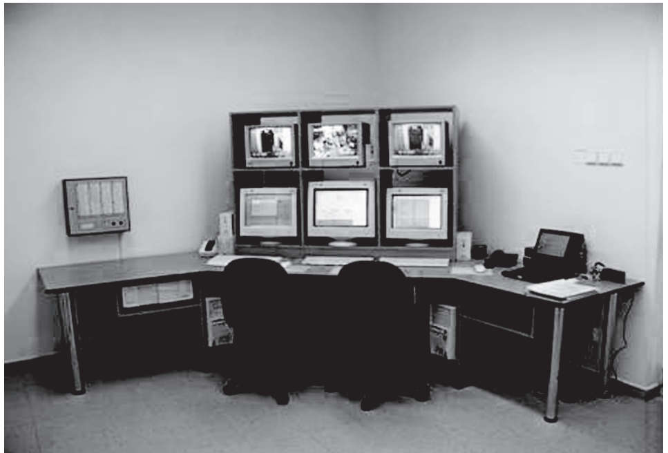
Figure 3: Upgraded Alarm Display and Closed Circuit Television Monitors Inside a Central Alarm Station at a HEU Research Reactor
