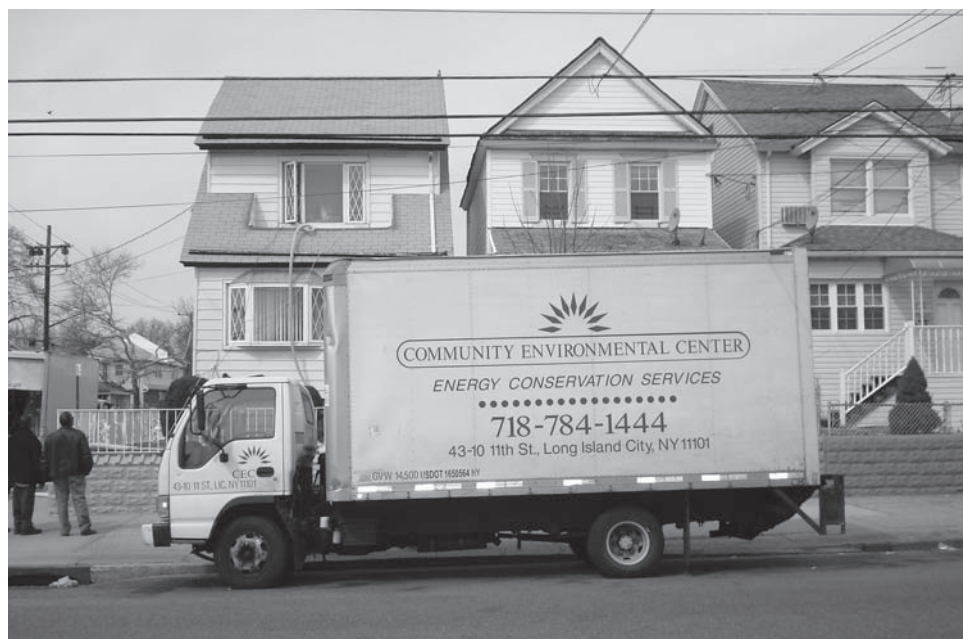
Figure 4: Community Environmental Center Workers Insulate a Home Being Weatherized in Brooklyn, New York
