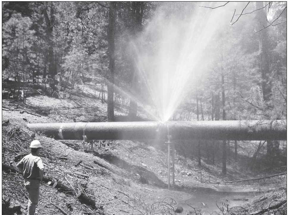
Figure 2: Existing Pipeline to be Repaired as Part of the Town of Payson’s Recovery Act-Funded Drinking Water Project
