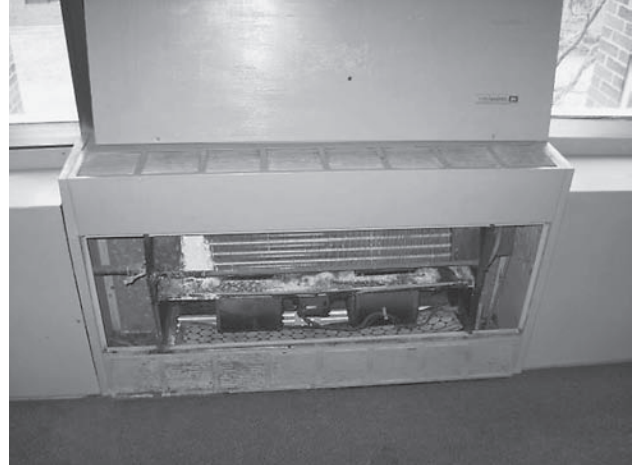
Heating unit to be replaced
