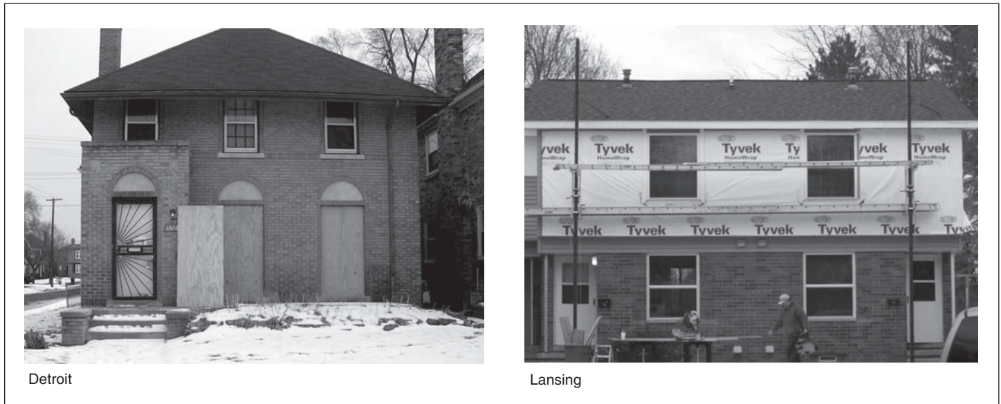
Figure 2: Photos of a Detroit Single-Family Home and Units at a Lansing Housing Complex That Are in the Process of Being Renovated with Recovery Act Funds
