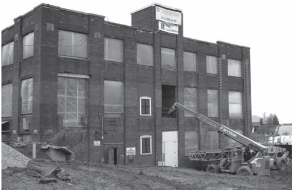
Hopewell Courtyard (renamed Westminster Place at Stewartstown) factory building being converted to living space.
