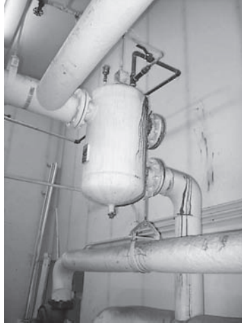
Boiler to be replaced
