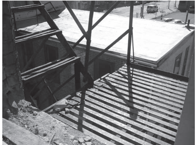
A fire escape at Greystone Apartments that the project will replace as part of safety improvements.
