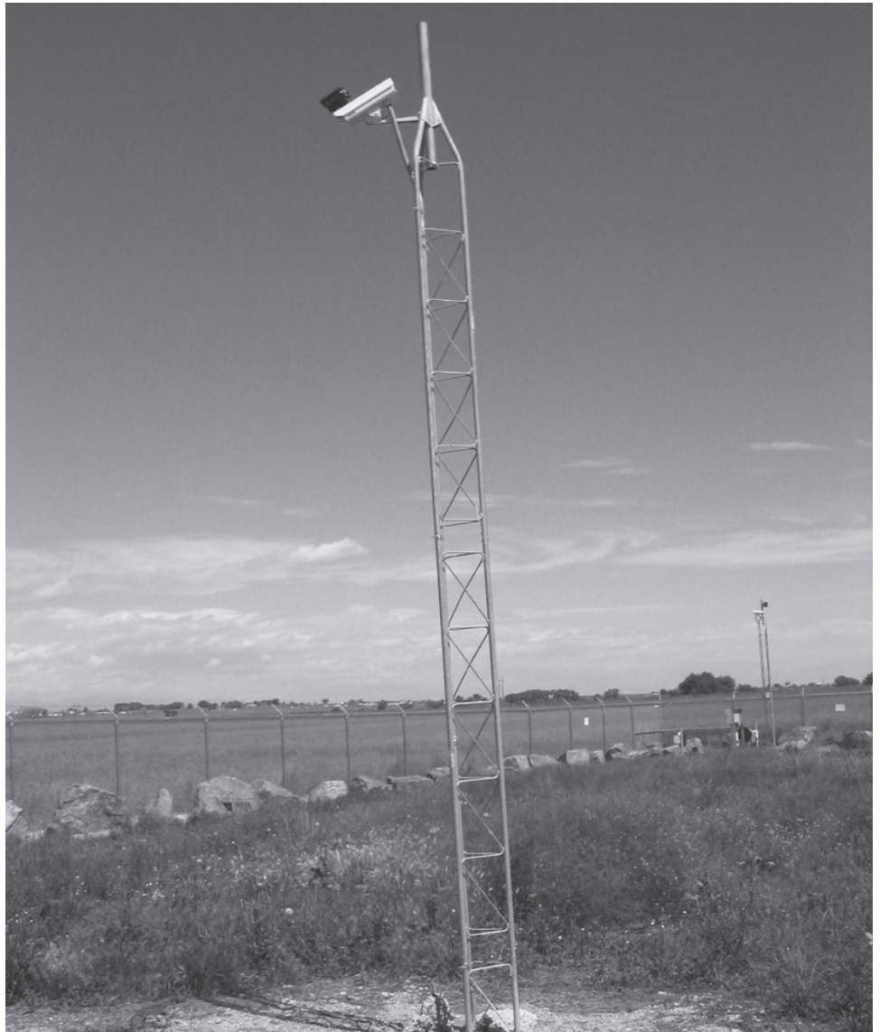
Figure 7: One of Many Closed-Circuit Television Cameras Installed at a Critical Facility
