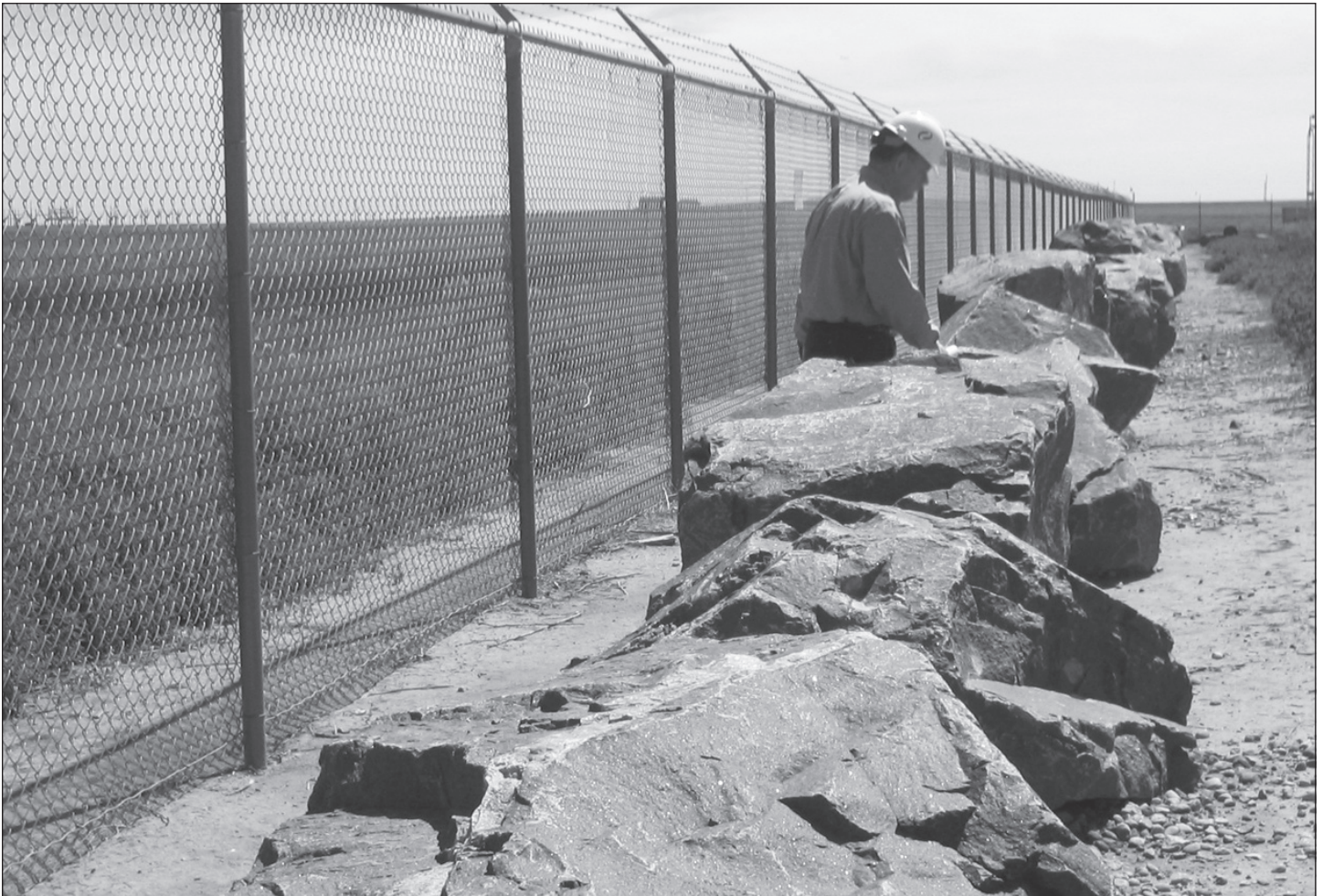
Figure 6: Boulders Installed inside Perimeter Fencing at a Critical Facility Serve as a Vehicle Barrier
