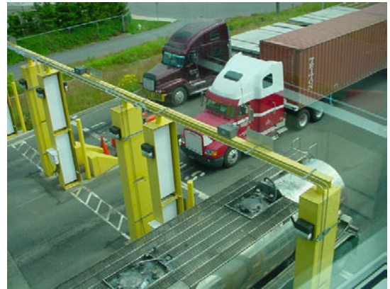
Portal monitors in use at the U.S. POE in Blaine, WA. Source: GAO.
