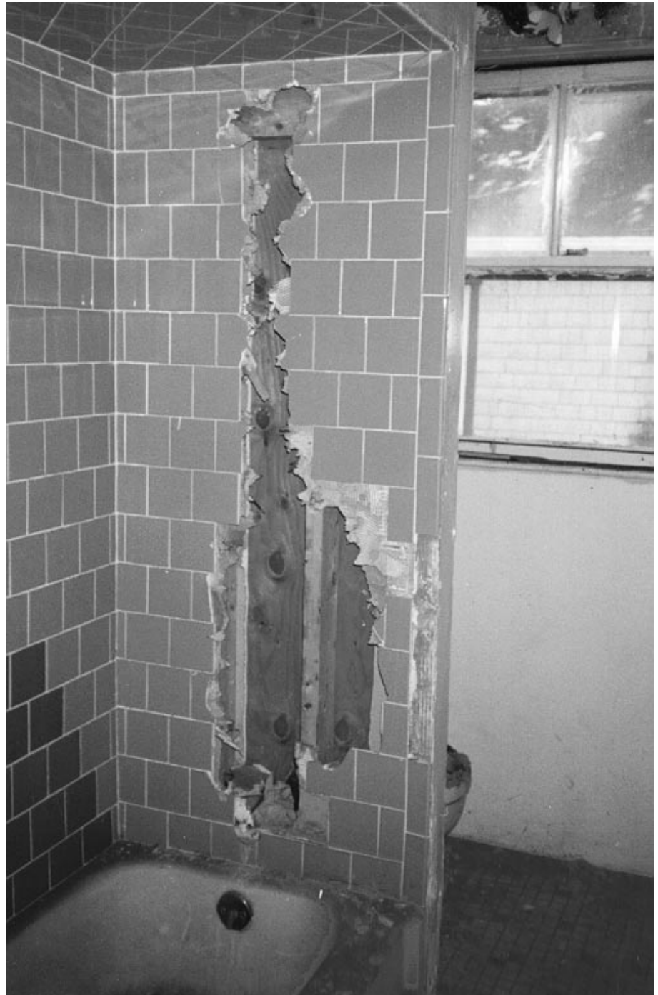
Figure 2: Copper Piping Ripped Out of Wall at an Improperly Secured Property
