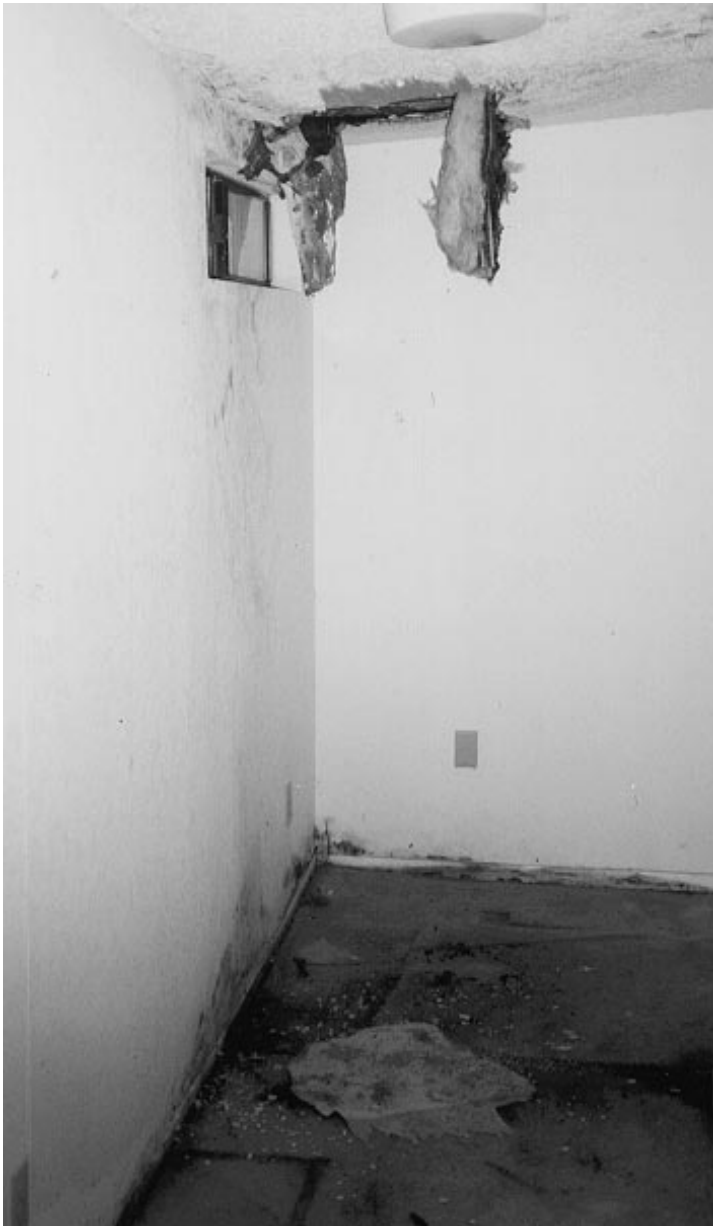
Water damage resulting from active roof leaks
