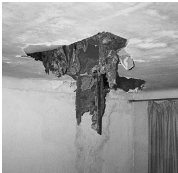
Significant water damage at a custodial property
