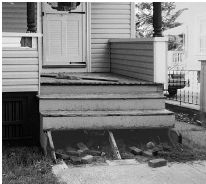
Broken stairs leading to property's front entrance
