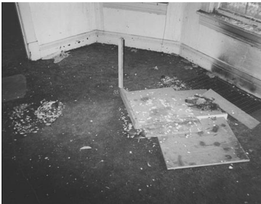
Dead and rotting pigeons, and bird droppings, at another custodial property
