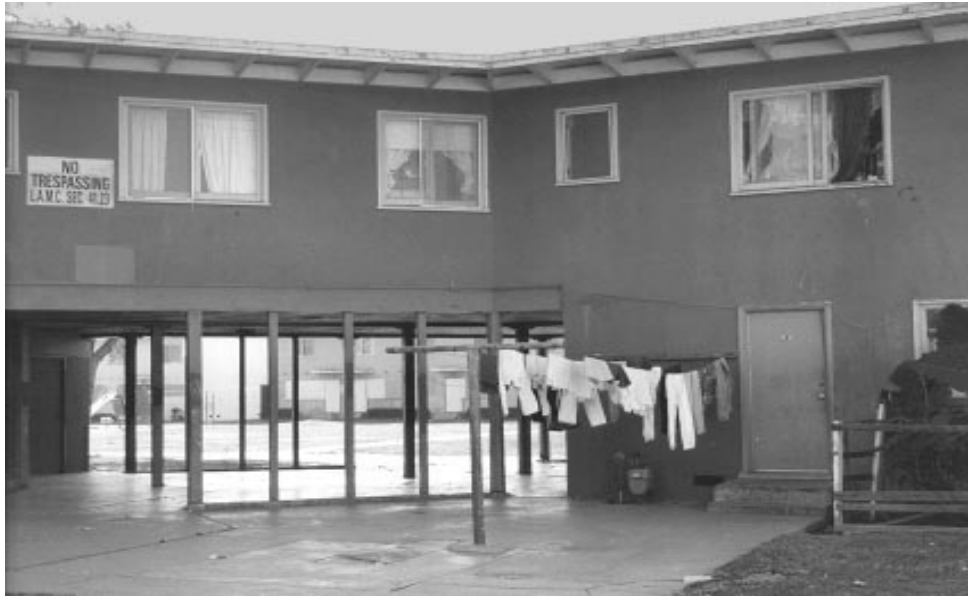
Dangerous entryway into original courtyard
