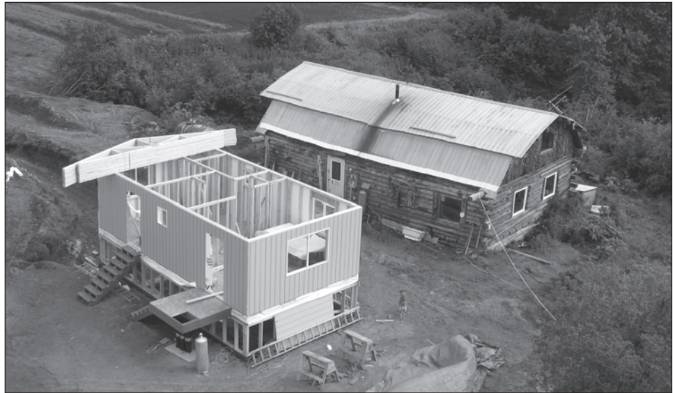
Figure 6: Small Grantee Replacing a Log Cabin with a 400 to 500 Square Foot Home Using $30,000 in IHBG Funds (ONAP Alaska Region)
