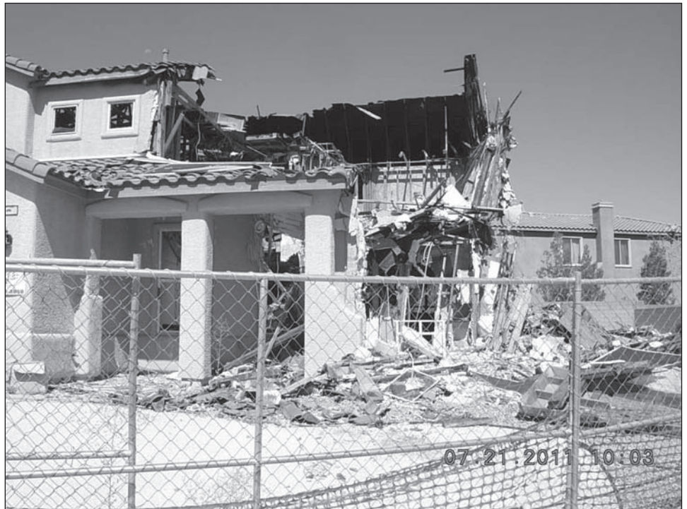
Figure 9: Damaged Property in Henderson, Nevada
