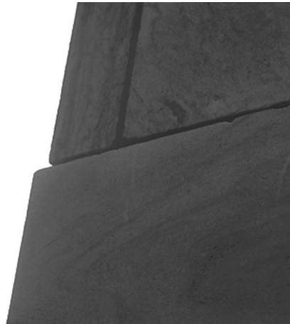
Figure 6: Stone Displacement Due to Effects of Age
