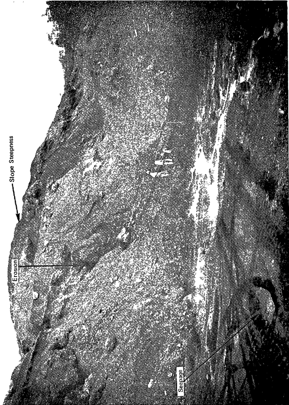
EROSION, SEEPAGE, AND SLOPE STEEPNESS PROBLEMS IDENTIFIED AT WASTE DISPOSAL SITE WE VISITED
