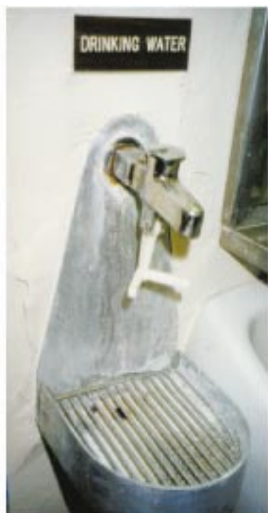
Corroded drinking water facility and damaged wall
