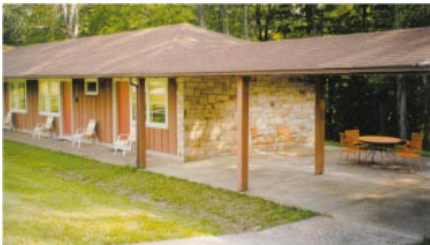
Figure II.7: Needed Exterior Repairs at Mammoth Cave Lodge
