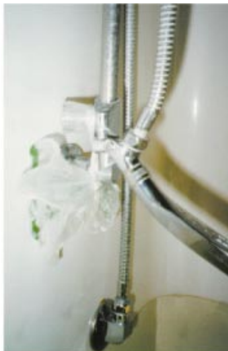
Plastic bag holding broken shower facility
