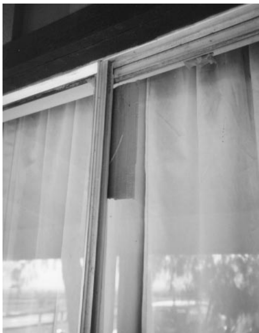
Duct tape on broken window
