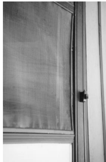
Broken handle and screen on back door
