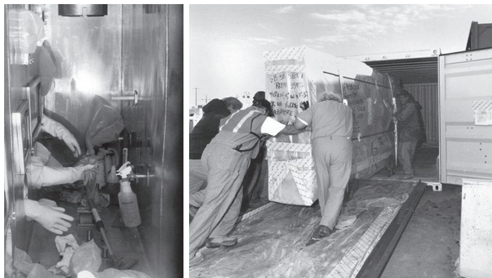
Figure 2: Workers Use Cerium Nitrate to Decontaminate a Glovebox; Workers Load a Dismantled Glovebox into a Shipping Container
