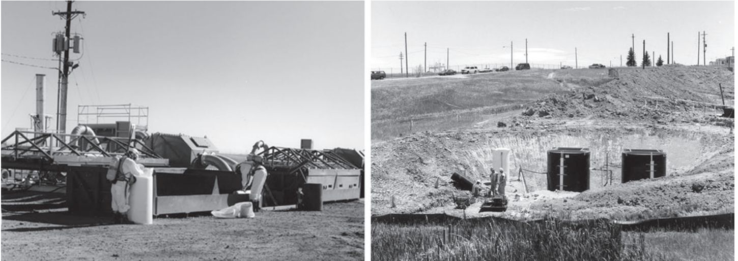
Figure 12: Treatment of Contaminated Soils by Thermal Desorption; Installation of a Passive Treatment System at the Mound Storage Site, Rocky Flats
