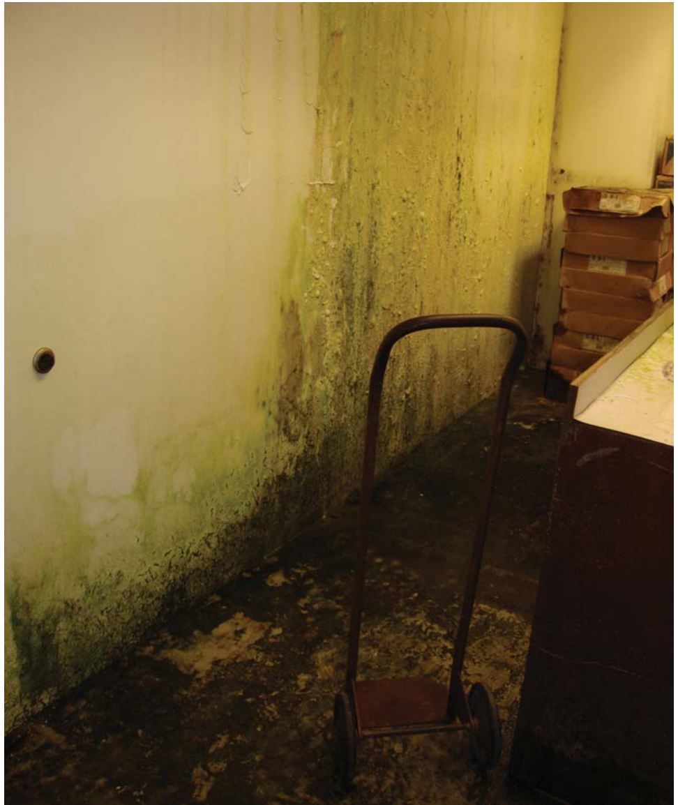
Figure 6: Rota Health Center Loading Area with Significant Mold
