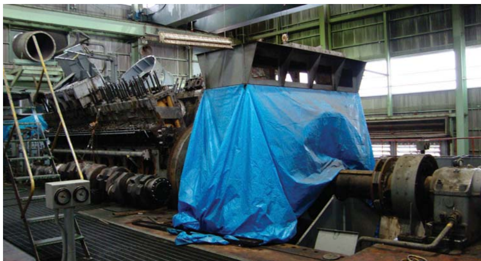
Figure 5: An Unused Saipan Power Plant Engine
