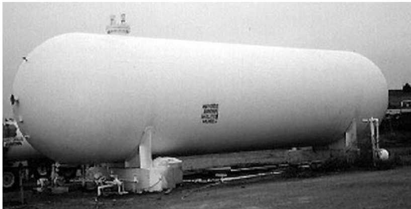
At the dealerships, the anhydrous ammonia is stored in pressurized "bullet" tanks. This bullet tank holds 30,000 gallons (about 77 tons).
