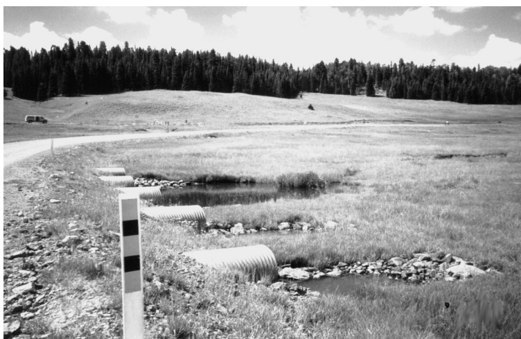
Road improvement to reduce steambank erosion. Multiple culverts employed to divert and slow flow.
