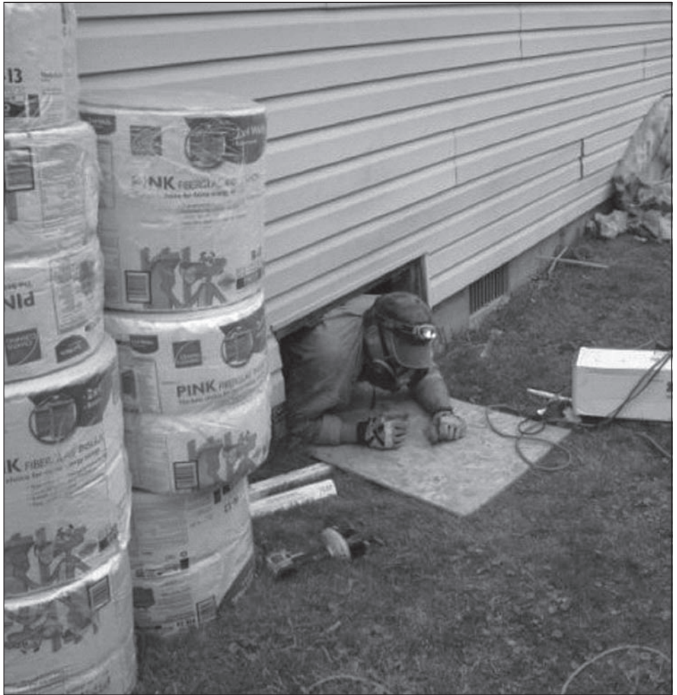
Figure 3: Contractor Installing Foundation Insulation in Hazel Park, Michigan Under the Recovery Act-Funded Weatherization Assistance Program
