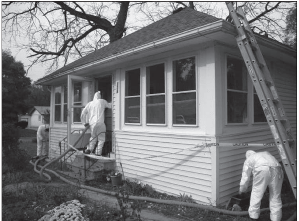
Figure 2: Contractors Installing Side Wall Insulation in Jackson, Michigan Under the Recovery Act-Funded Weatherization Assistance Program
