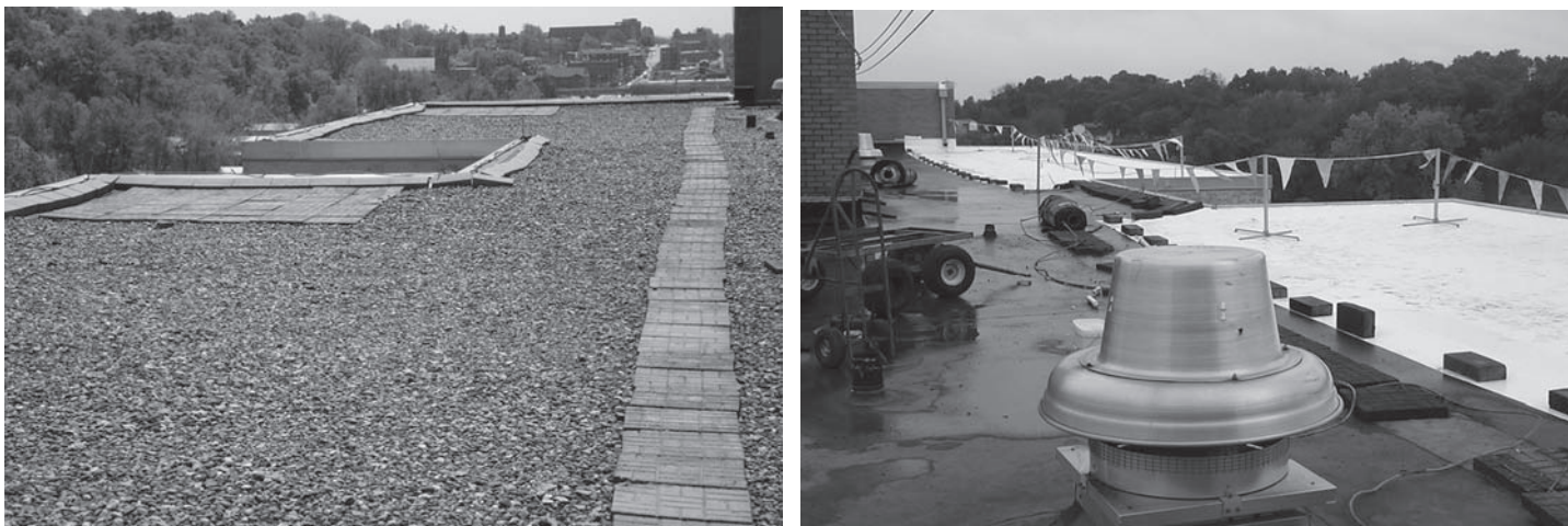
Figure 3: Roof Repairs to an Iowa Public Housing Facility, before Work Began and Work in Progress
