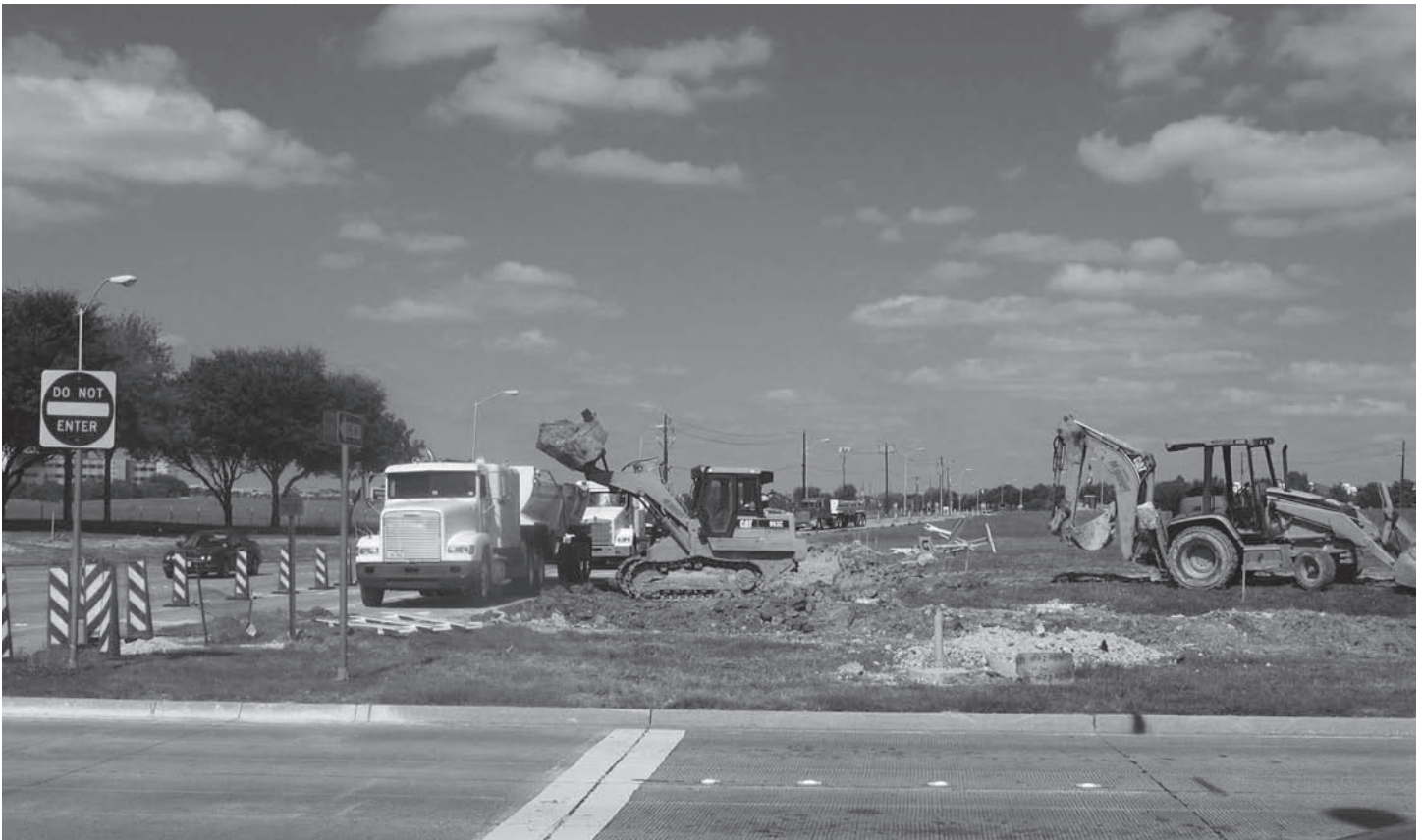
Figure 4: Improvements in Progress at Intersection of Preston Road and Legacy Drive in Plano, Texas
