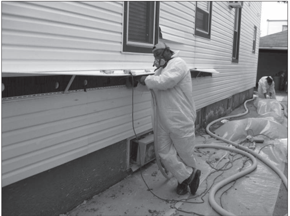
Figure 3: Community Environmental Center Workers Insulate a Home Being Weatherized in Queens, New York
