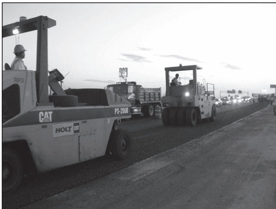
Figure 6: Fort Worth, Texas, Interstate 820 Resurfacing in Process to Repair Roadway Deterioration Using Recovery Act Funds
