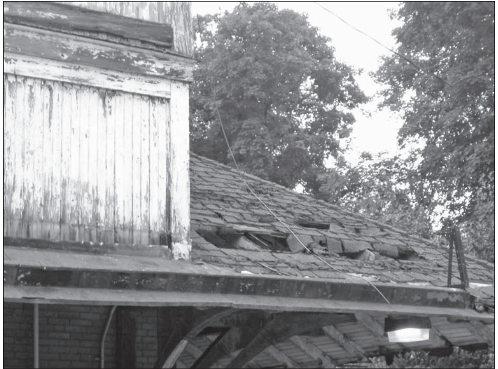
Figure 2: Holes in the Roof of SEPTA's Tulpehocken Station That Will Be Repaired Using Recovery Act Transit Capital Assistance Funds
