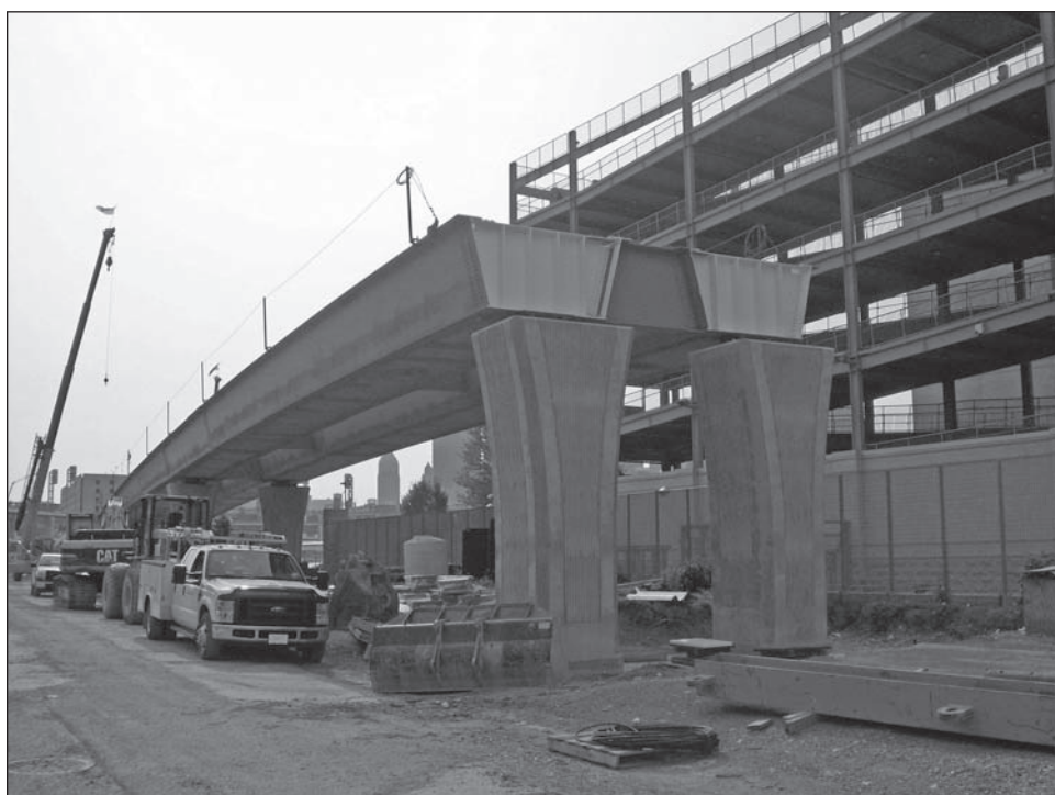
Figure 5: Steel Girders for the Port Authority's North Shore Connector Project, Near New Allegheny Avenue Station, Which Will Be Funded by Recovery Act Money
