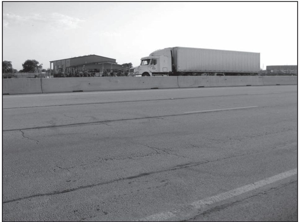
Figure 5: Fort Worth, Texas, Interstate 820 Roadway Deterioration Prior to Resurfacing Using Recovery Act Funds
