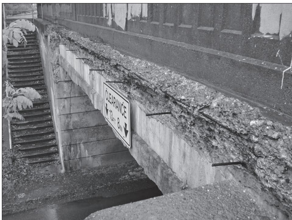
Figure 3: Rail Bridge on SEPTA's Lansdale Regional Rail Line That Will Be Rehabilitated Using Transit Capital Assistance Recovery Act Funding
