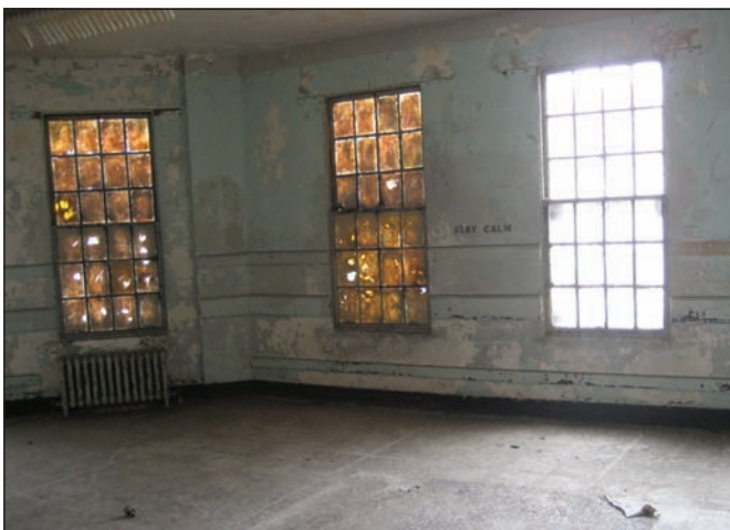
Yellowed windows, asbestos on the wall, peeling paint, and floor panels breaking off, West Los Angeles, Calif.
