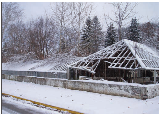
Greenhouse roof is deteriorating and has several broken windows, Marion, Ind.
