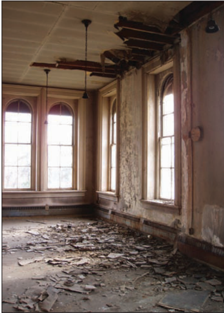
Deteriorating ceiling and wall, Dayton, Ohio
