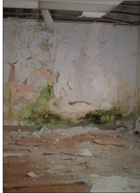
Signs of mold and asbestos on the wall of a vacant building, Marion, Ind.
