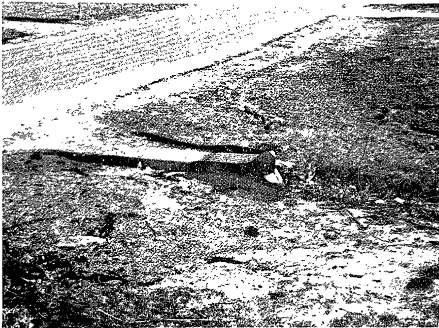
STORM WATER DAMAGE TO HOMEOWNER'S FRONTYARD.
