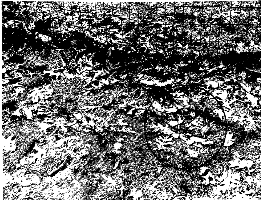
HOME C.— CIRCLED AREA IS EXPOSED CORNER OF ABSORPTION BED. WHEN THE TOILET IS FLUSHED, WATER FROM THE SYSTEM PERCOLATES TO THE SURFACE AND RUNS DOWN THE SLOPE OF THE YARD.
