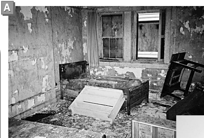
Figure 3: Deteriorating Conditions at St. Elizabeths
