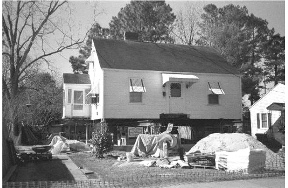
Figure 3: House in North Carolina in the Process of Being Elevated to Mitigate Flood Damage
