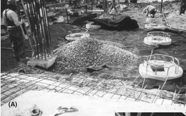
(A) Shows the bentonite membrane and various layers of material under the slab. The bentonite absorbs any water that passes by the filtering system. When the bentonite gets wet it becomes sticky and gooey, thus sealing everything.
