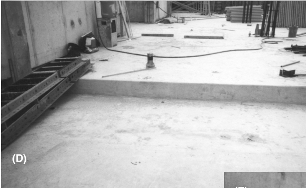
(D) Shows inside the computer room area looking towards the southeast side of the building, with the 12-inch recessed slab in the computer area where the raised floor is to be installed.
