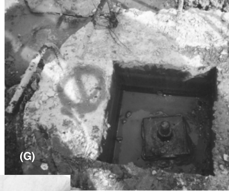
(G) Shows a typical auger cast stressed, torqued, and locked pile cap, which is a structural system installed to prevent the building floating as a result of the buoyancy force from the hydrostatic pressure of flood waters.
