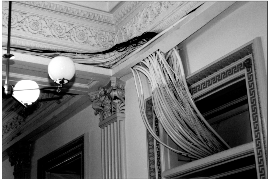
Figure 6: Unsightly Bundles of Wires in an EEOB Hallway
