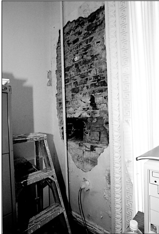
Figure 4: Extreme Water Leak Precludes Replastering Wall in a 3rd Floor EEOB Office
