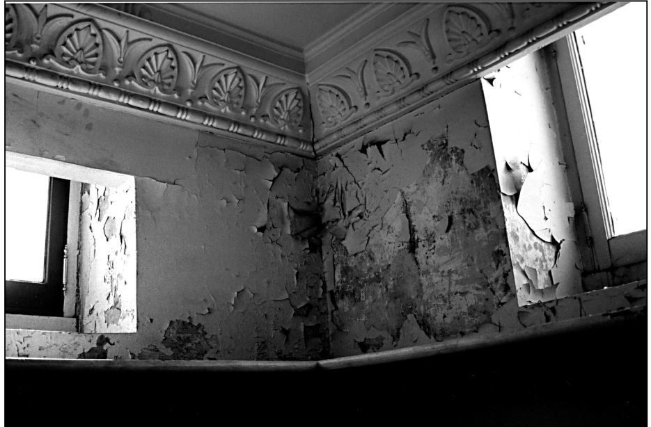
Figure 5: Deteriorating Interior Wall Due to Water Damage in an EEOB Historic Library
