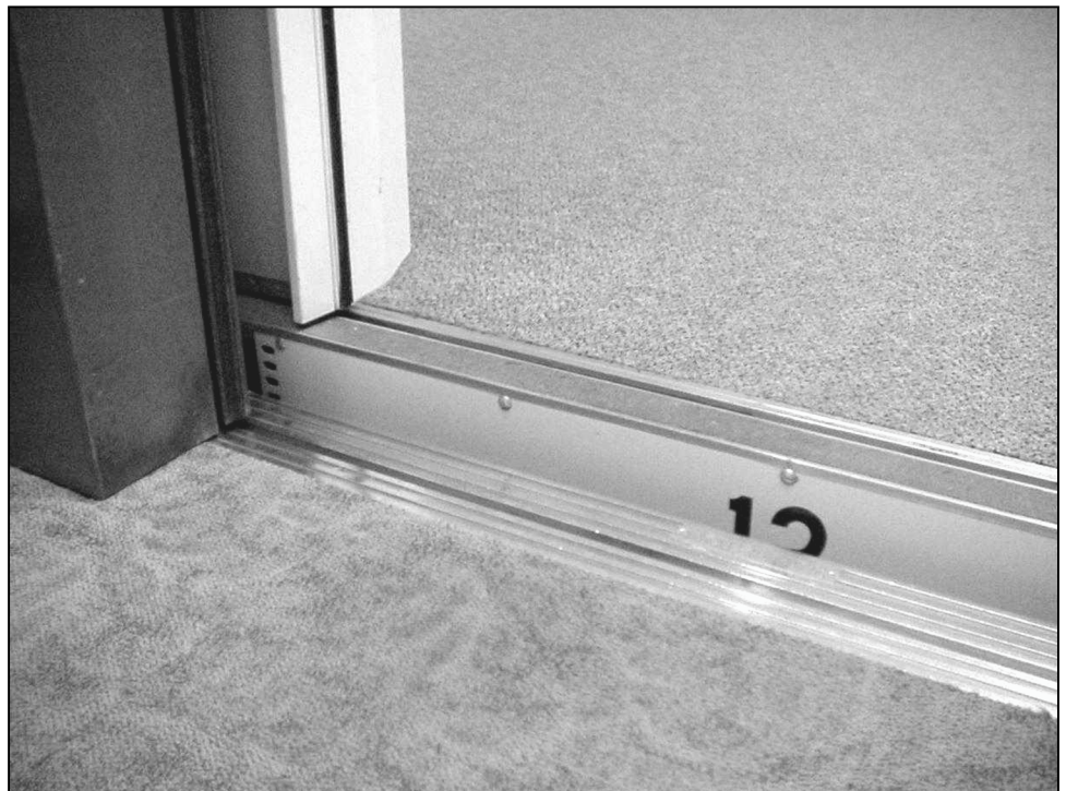
Figure 7: A Problematic Elevator in the Jackson Federal Building
