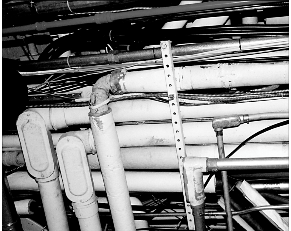
Figure 3: Cluttered Basement Ceiling in EEOB With Steam and Water Pipes Dangerously Close to Electricity
