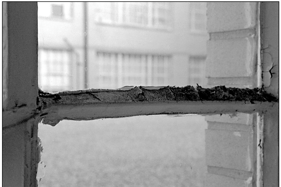
Figure 2: Window With Peeling and Chipping Paint in a First Floor FOB 3 Office
