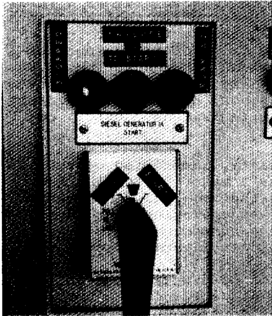
Operators make extensive changes to board labeling.
