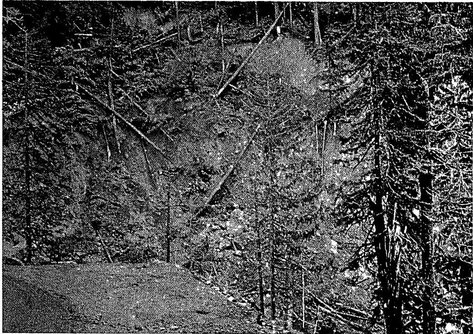
5 Earth slide on BLM road construction project
